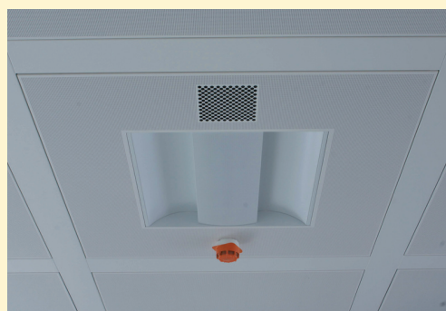
The ceiling designed for a major refurbishment project in Dublin combines cooling with other services such as lighting and smoke detectors into a zone just 85 mm deep.
