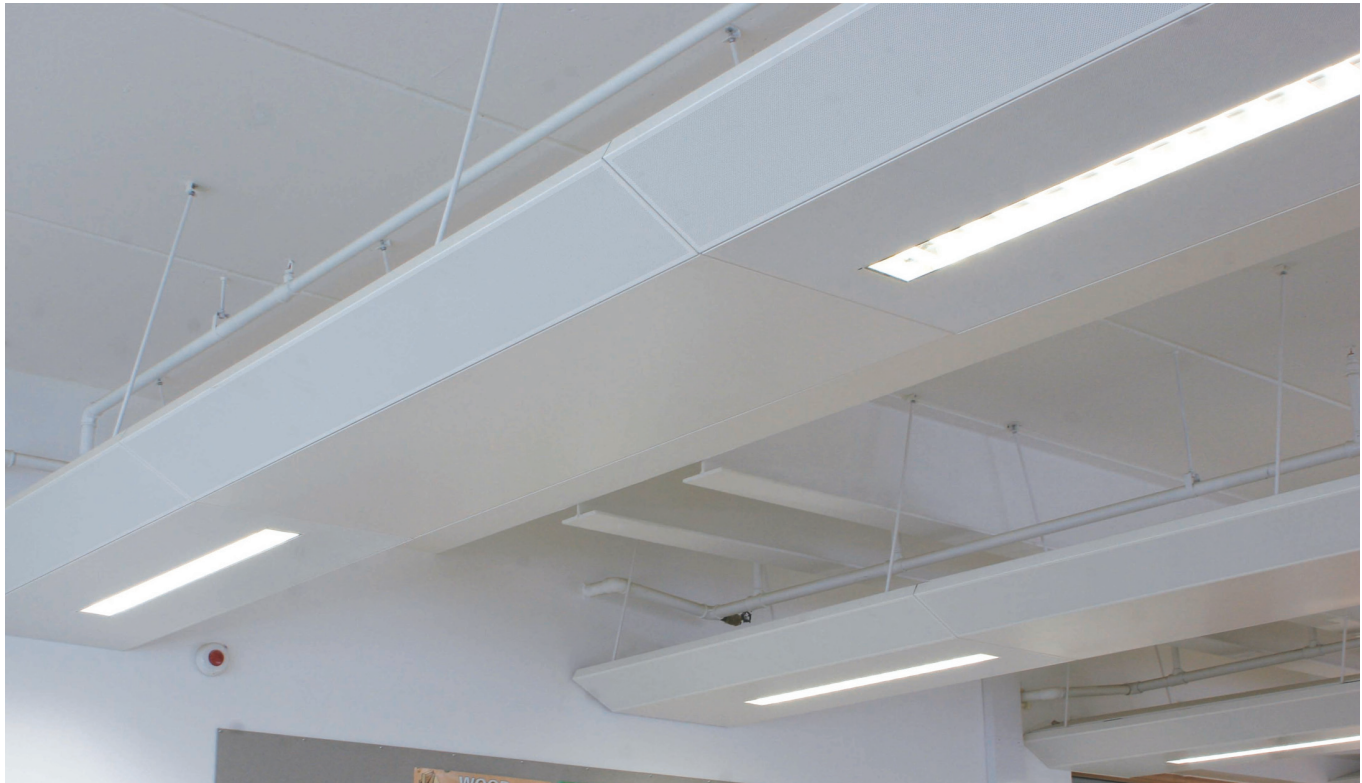
Figure 2: Suspended module including radiant heating, lighting and acoustic absorption material
