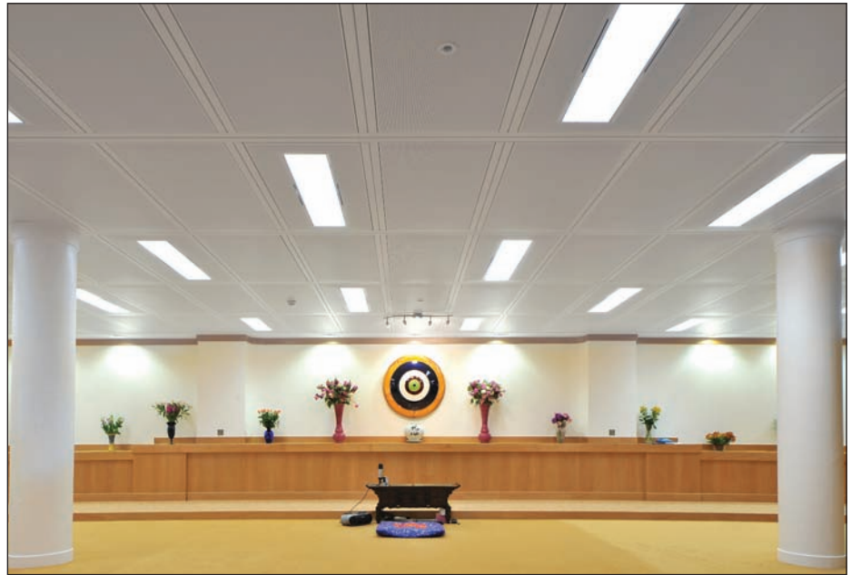
SAS’ radiant chilled ceiling was installed at a Queen Anne Street development in London.
