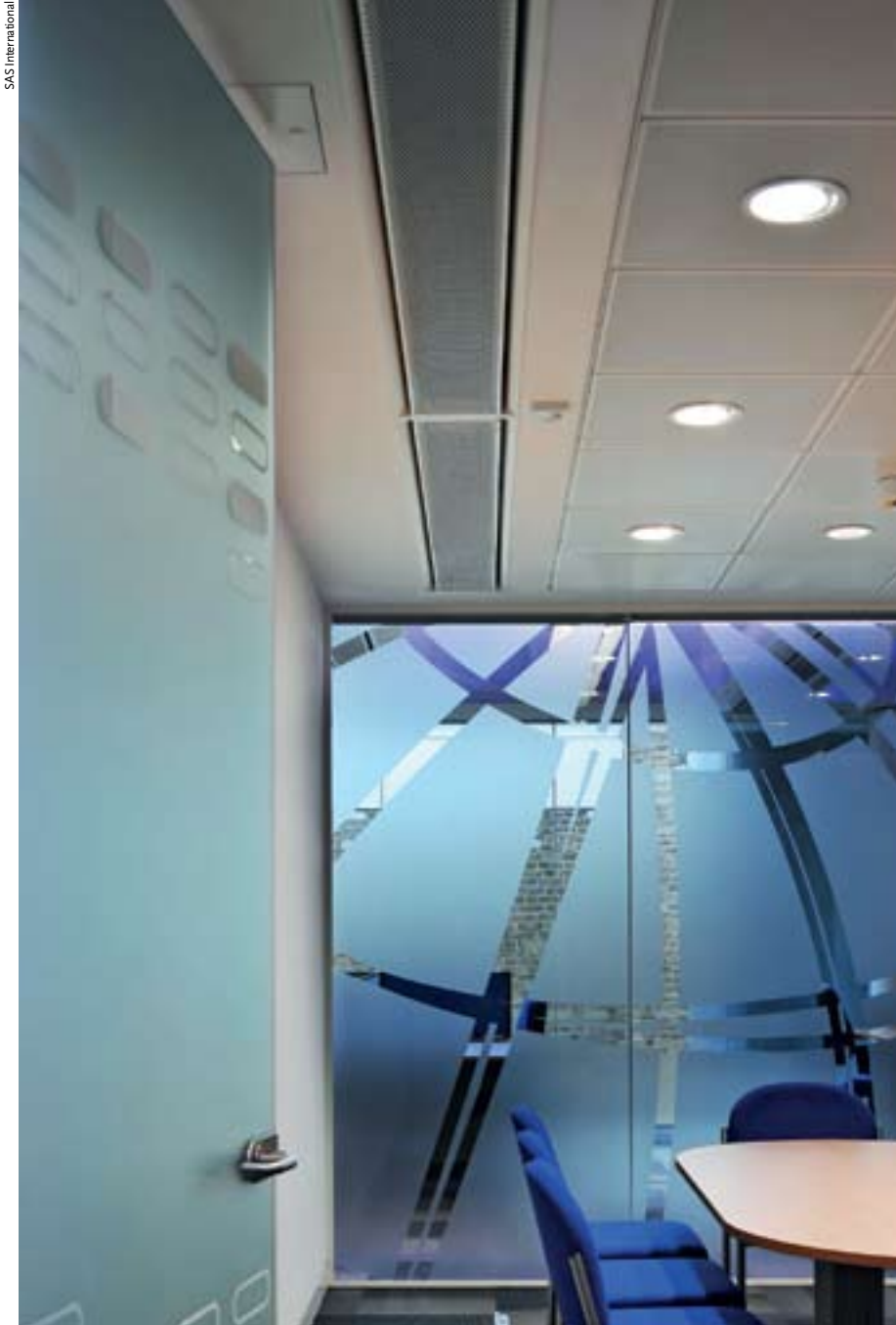
Cooling for the building is provided by chilled beams supplied by SAS International, which was part of the project team
